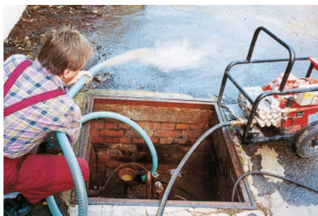
Draining of underground shaft with sludge pump - high-pressure water transports sludge away rapidly.
