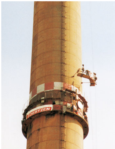
Paint removal of obsolete signage on 200 m high chimney with water-sandblasting system TORNADO and high-pressure unit E 320 - even with 150 m height still 285 bar at the nozzle.
